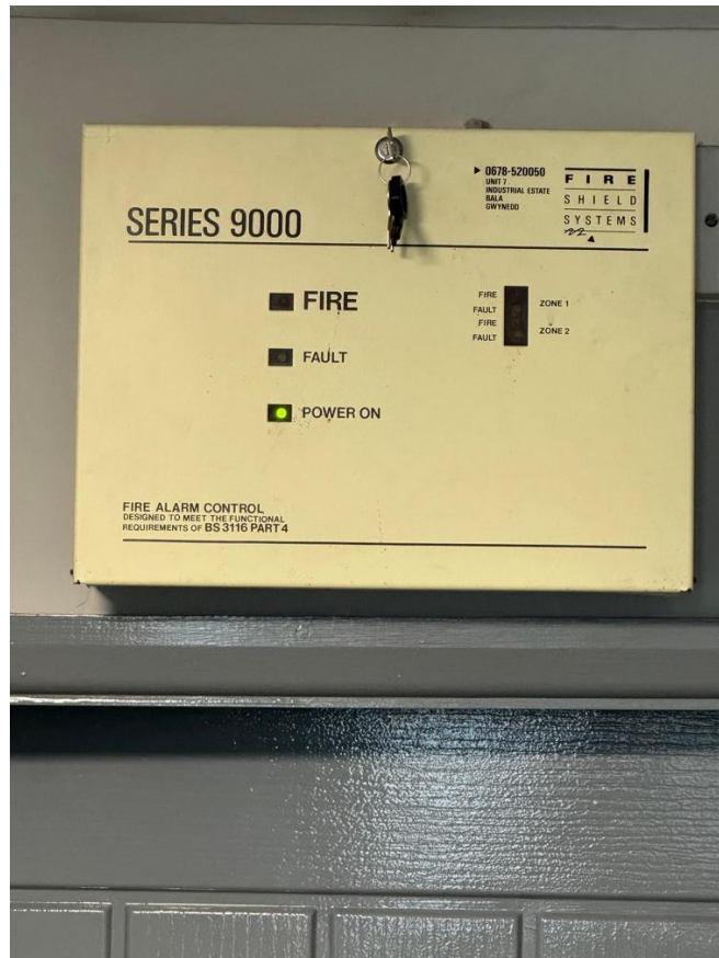
Fire alarm control unit position in front lobby of building
